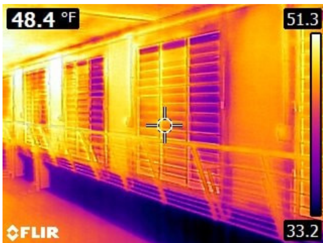
Above FLIR photo was taken at a 2,400 head finishing site in eastern Iowa when the outside temperature was below 0° F temperatures.
